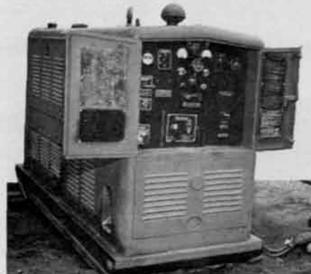
Figure 1—Diesel Generator RD-14A.
